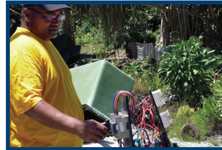
Tomasi Tafua, General Manager of Energy, explains how the solar generated power is converted to electricity in the pilot renewable energy project, supported by UNDP, in Fakaofu, Tokelau. @ UN/Ariane Rummery
